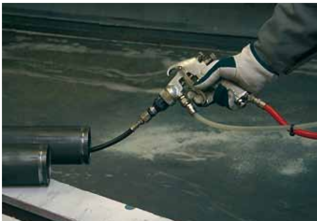
Piping modules are protected with oil in order to prevent corrosion during transportation and storing.
