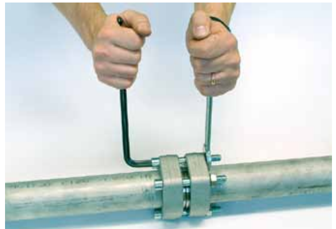
The greased bolts (and nut) are tightened to the given torque to complete the installation.
