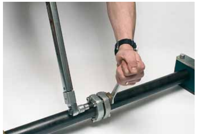
The greased bolts (and nut) are tightened to the given torque to complete the installation.
